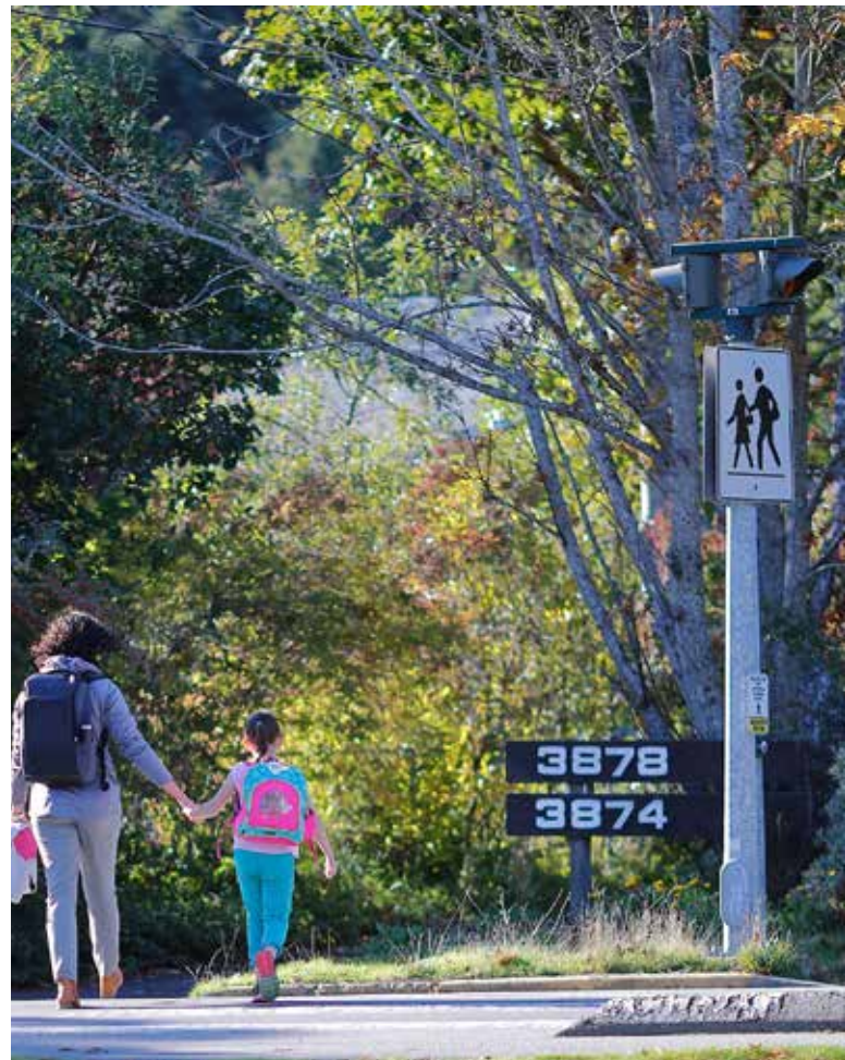
Pedestrian activated solar crossings.
