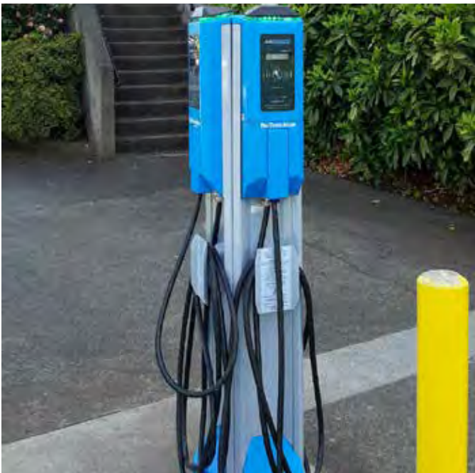
Public electric vehicle charger
