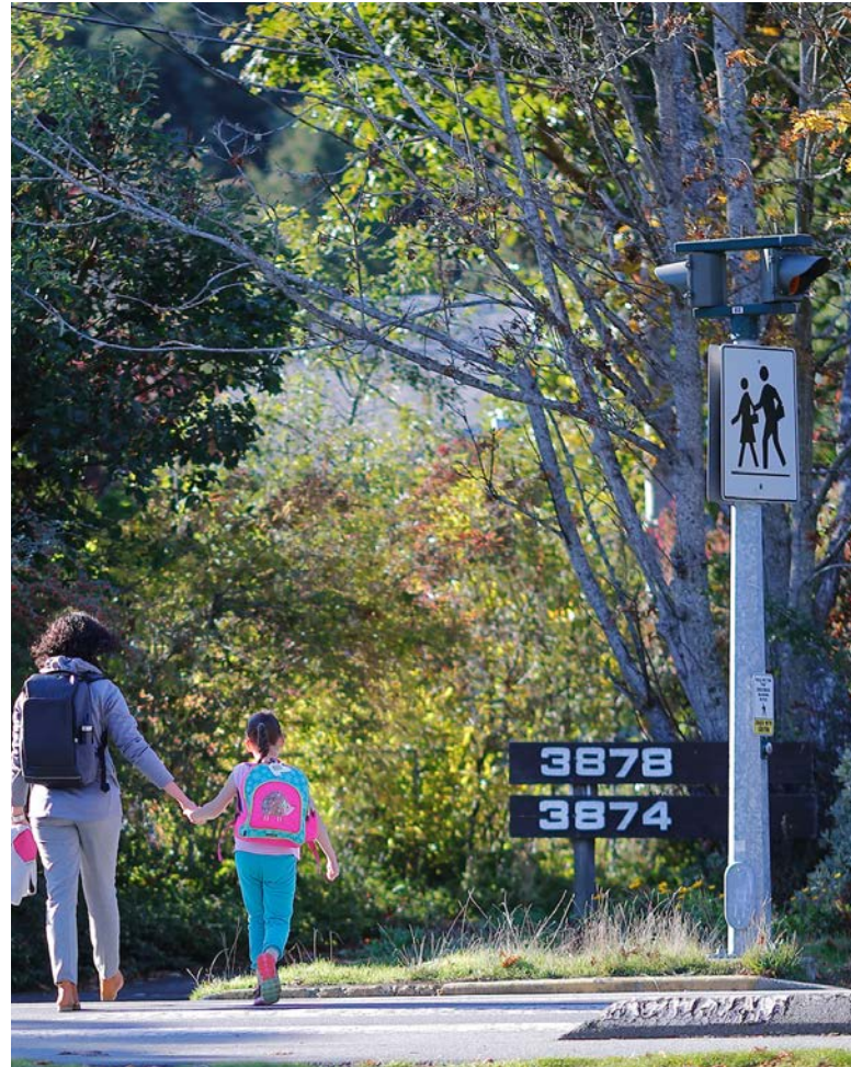
Pedestrian activated solar crossings.
