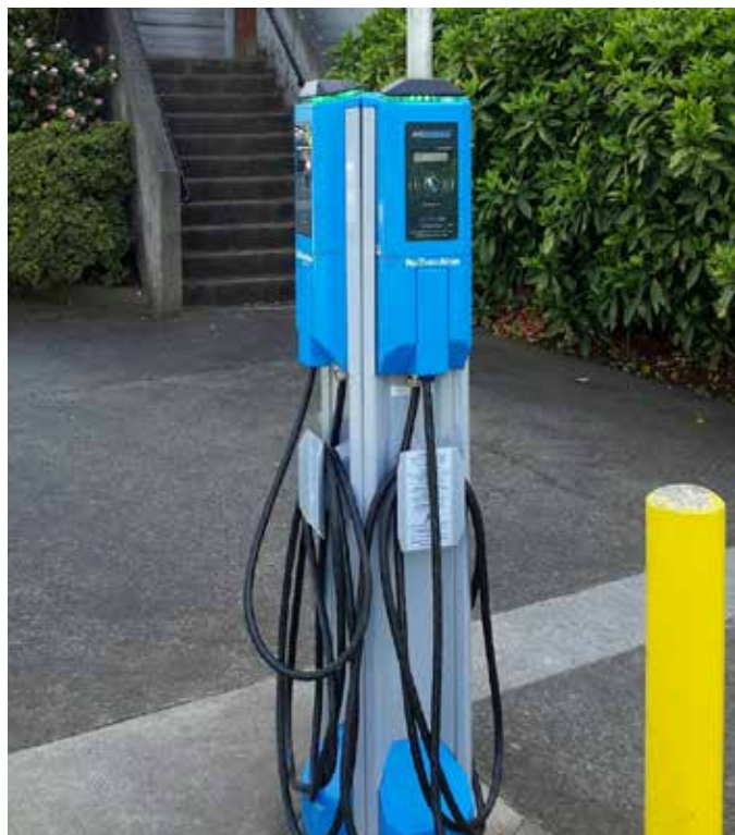
Public electric vehicle charger
