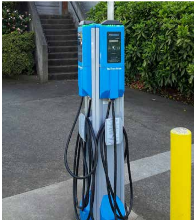
Public electric vehicle charger
