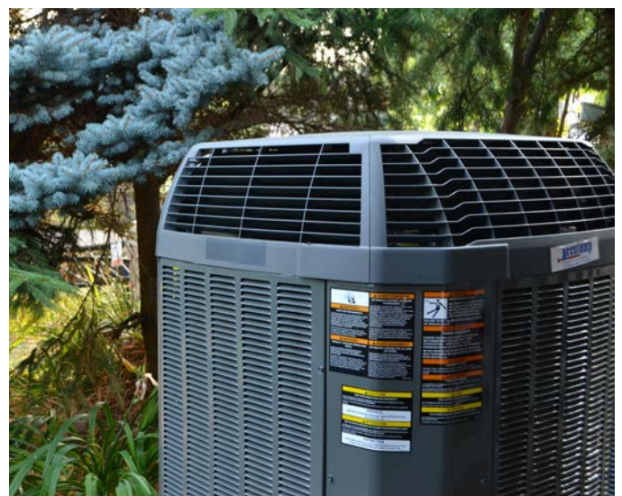
Electric heat pump
