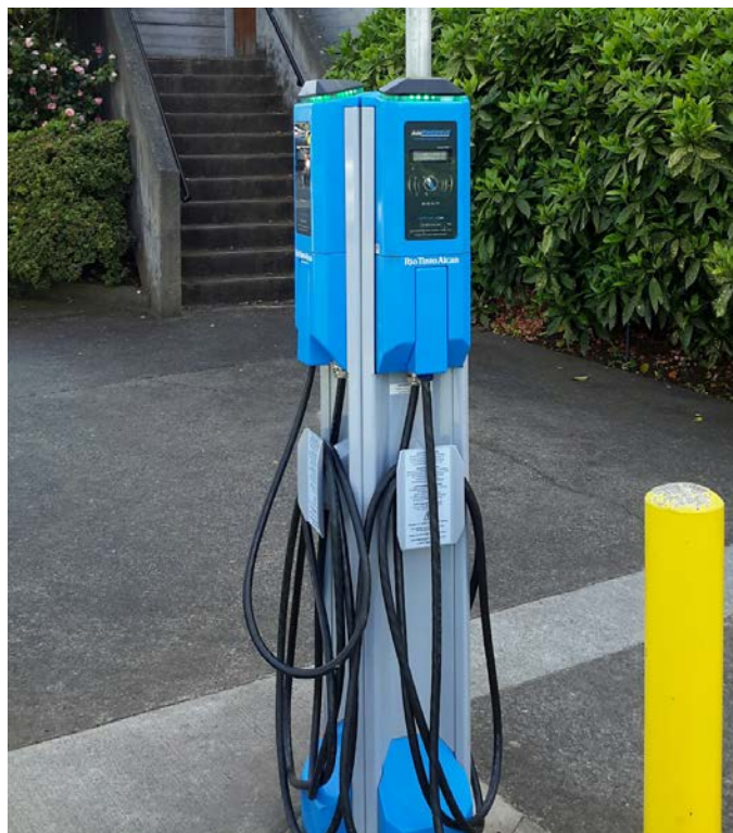
Public electric vehicle charger
