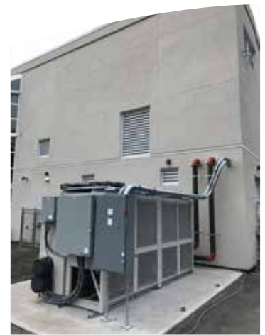
New air source heat pump installed at Gordon Head Rec Centre in 2017.
