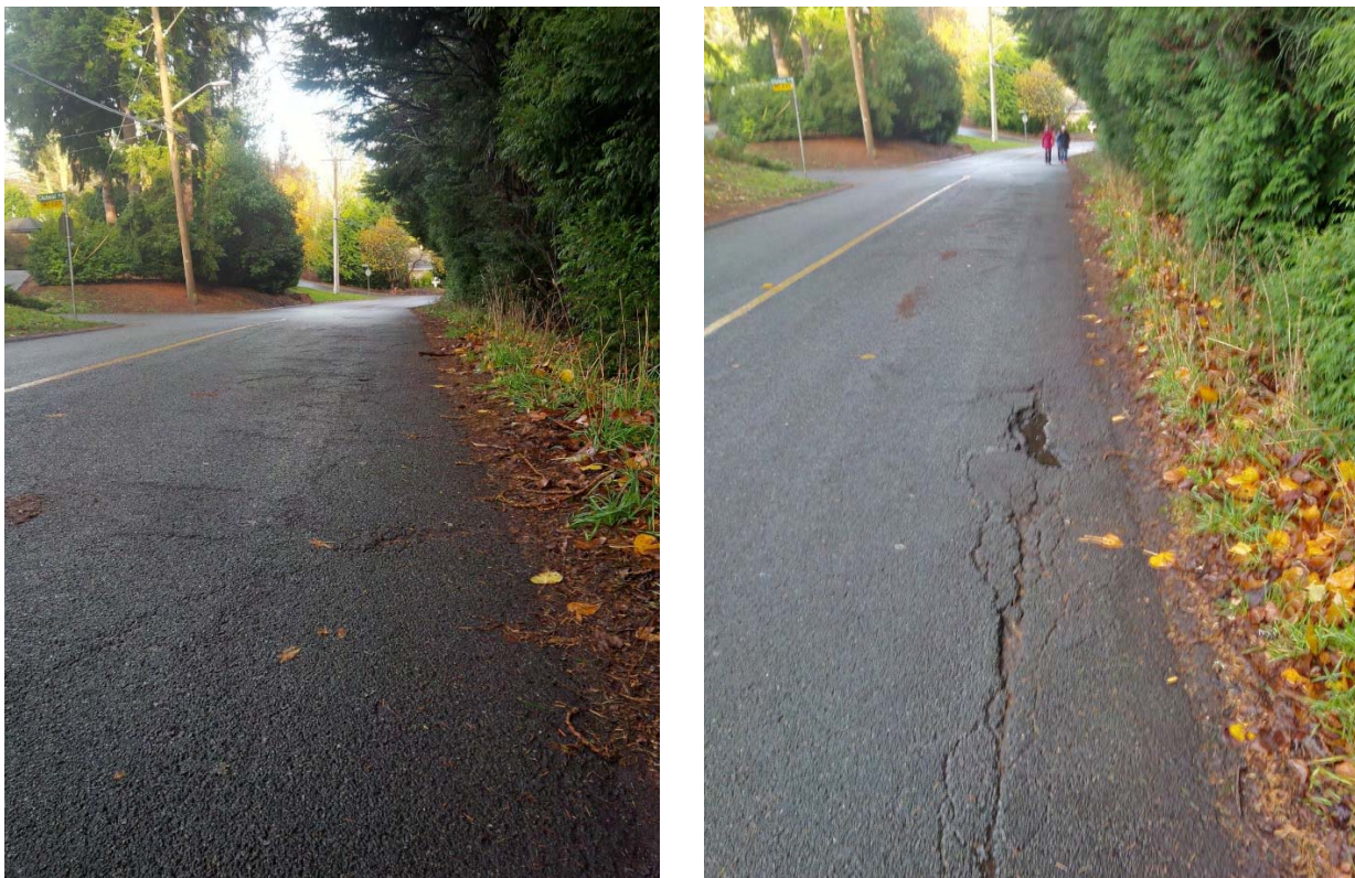
Figure 3: Road surface damage on Del Monte Avenue caused by Leyland Cypress roots
