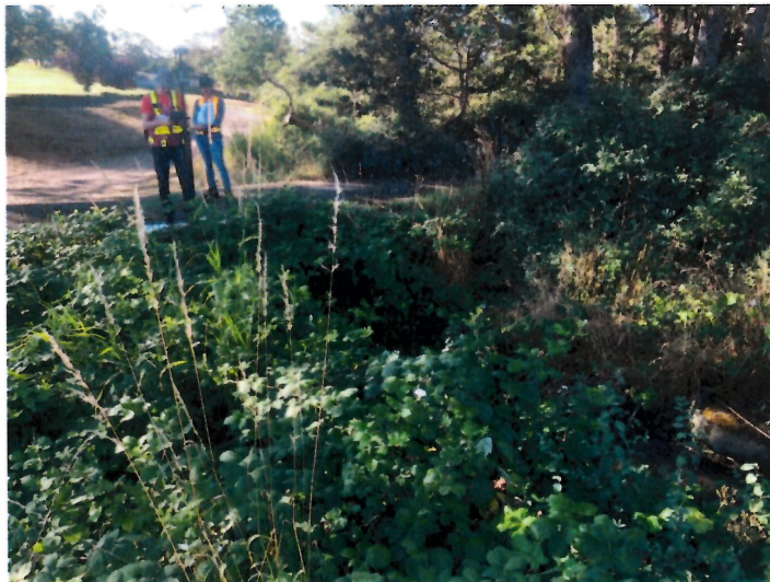
Photo 4: Creek channel gully and access path downstream of 4 th Hole Fairway. Note overgrown with invasive species.
