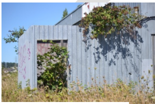
Mechanical Air Distribution Lean-to
